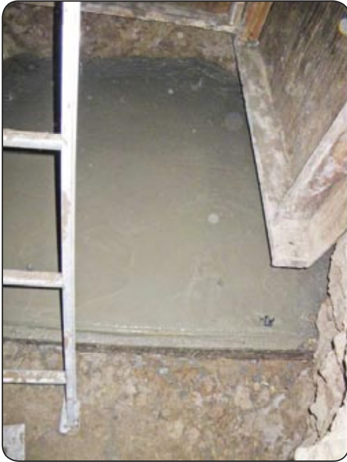
Concrete foundation at bottom of dig shaft. Also visible: some of the 2X4s and plywood that will be replaced by a stainless steel frame and high density polyethelene (HDPE) sheets.
